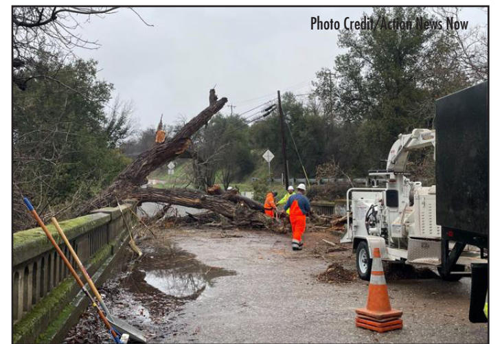
Crews work to remove the tree that fell on the Breckenridge Bridge
